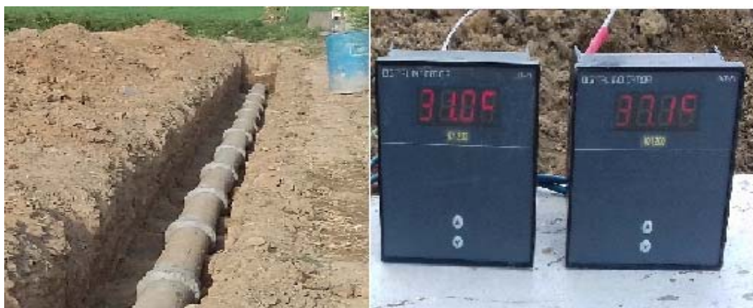
Fig 2. the buried pipes and temperature indicator used for study.
