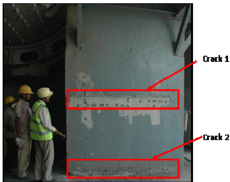
Fig.7: Elevation of cement mill foundation showing major crack position
